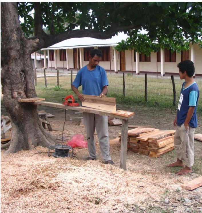
Nando making floor foundation boards. OLMC Primary School Zumalai is in the background.
